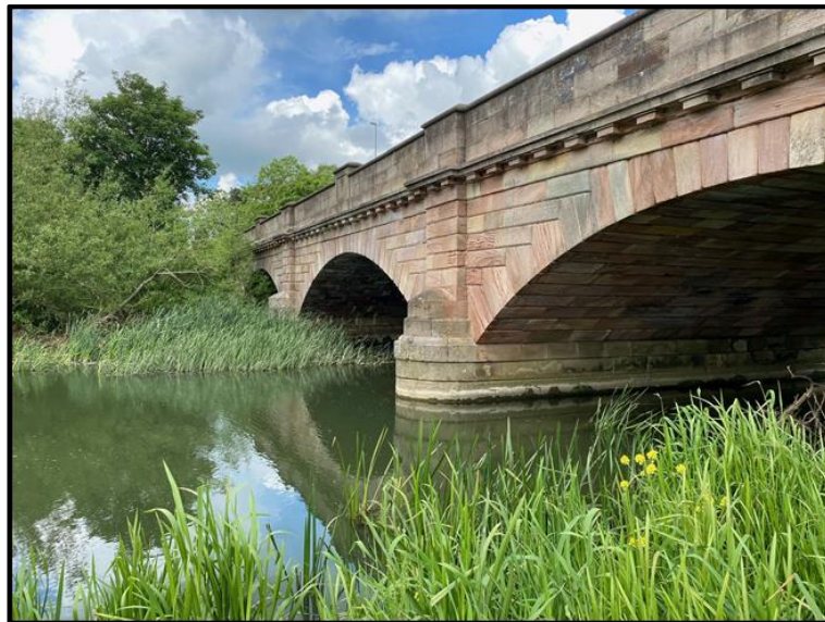
Figure 1-2 – Three arch bridge located further north on London Road, with one arch partially blocked by overgrown vegetation. Evidence of reduction in river flow capacity of the River Great Ouse.
