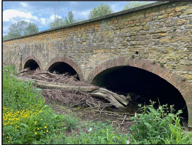
Figure 1-1 - Tombs Meadow Arches located on London Road (north of the High Street) partially blocked by debris.
