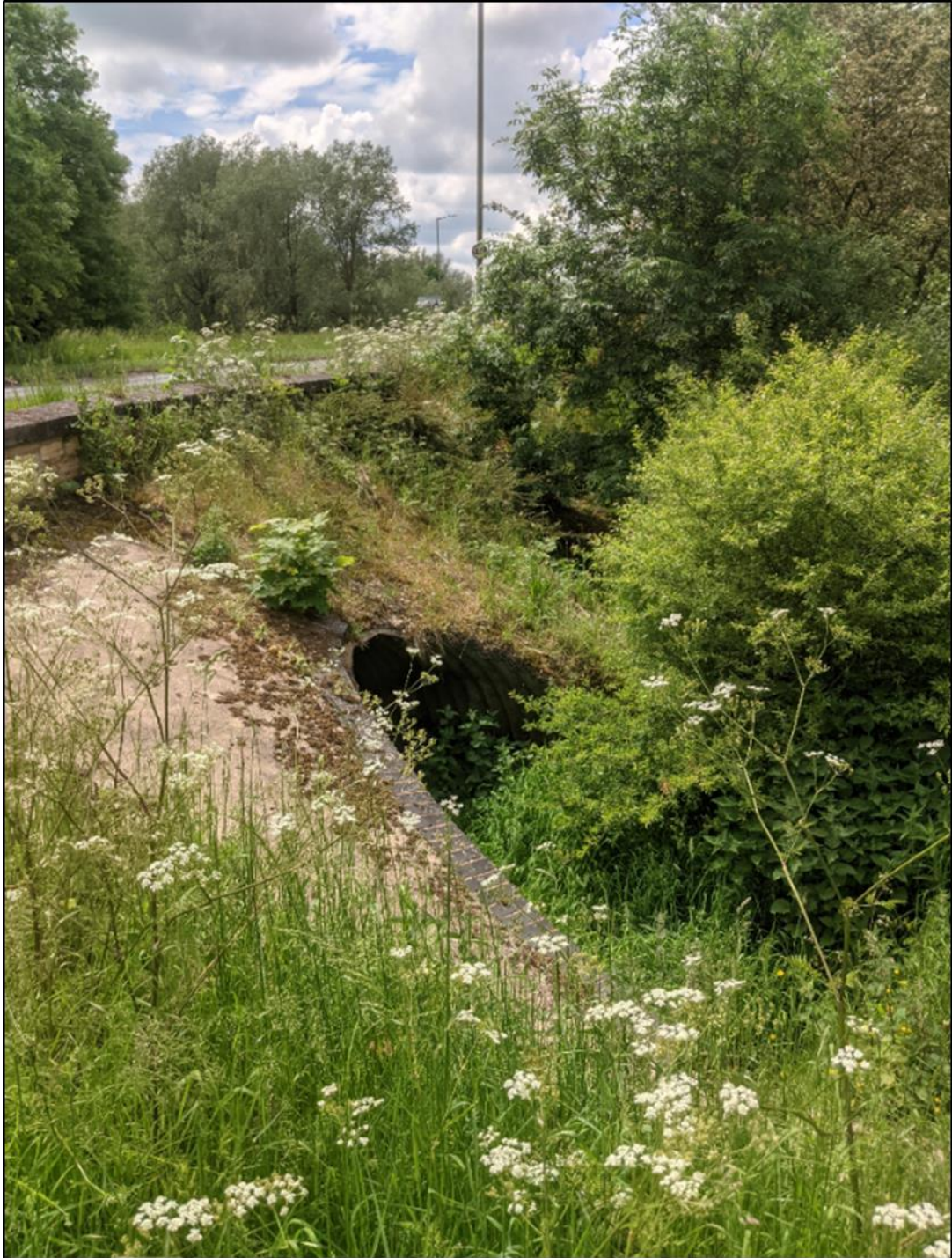
Figure 1-4 - Three culverts under Queen Eleanor Street. Evidence of at least two of the three culverts partially or totally blocked with debris and overgrown vegetation. Culverts potentially connected to River Ouse Valley Park.
