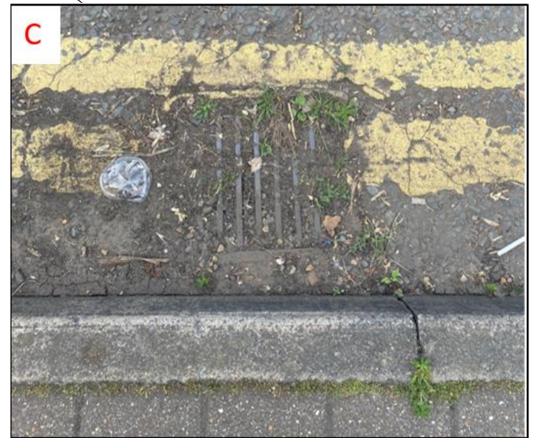
Blocked drain at Prospect Road which had the potential to exacerbate flooding during a storm event.
