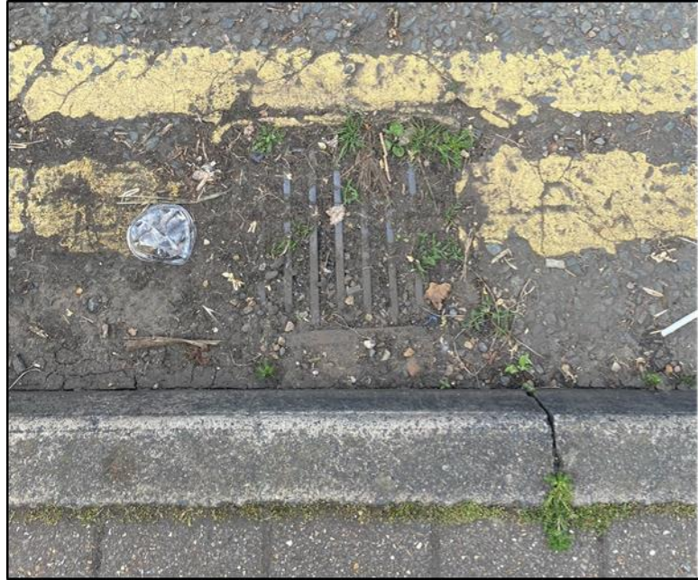
Figure 1-6 - Evidence of blocked drain at Willow Lane and Prospect Road.
