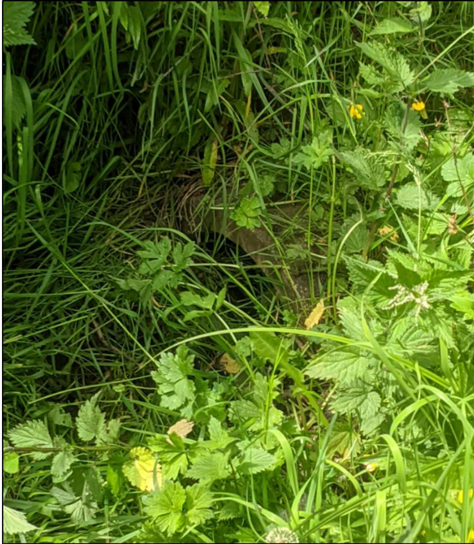
Figure 1-5 - Evidence of approximately 300mm culvert partially blocked with debris and vegetation. This culvert is connecting culverts in Figure 1-4 (culverts of significantly bigger dimensions and capacity) with the River Ouse Valley Park.
