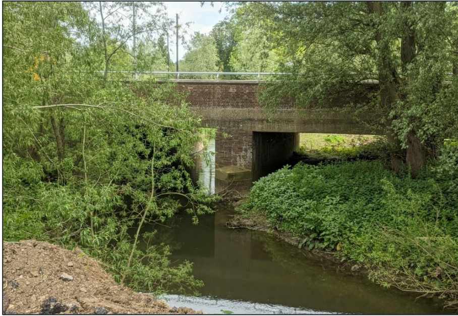
Figure 1-4 - Evidence of overgrown vegetation blocking one of the Watling Street bridge spans downstream of the River Ouzel. It might reduce the capacity of the bridge to convey river flows during extreme flood events.
