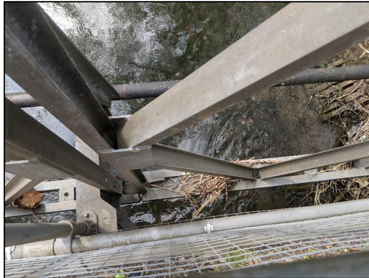
Figure 1-2 – Evidence of debris from a high flow event on a bridge downstream of the River Ouzel between the Bletchley Town Cricket Club and Watling Street.
