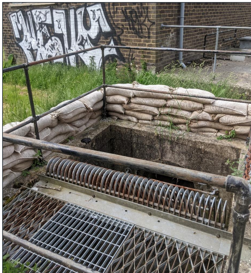
Figure 1-3 - Sandbags located between Bletchley Town Cricket Club and Watling Street, downstream of the River Ouzel.
