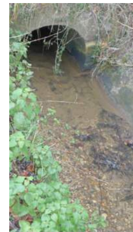
High St East Adjacent to site Sand in drainage tunnel
