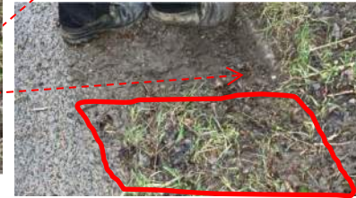
High St West Recovered Kerbside Road Loss to overgrown vegetation
