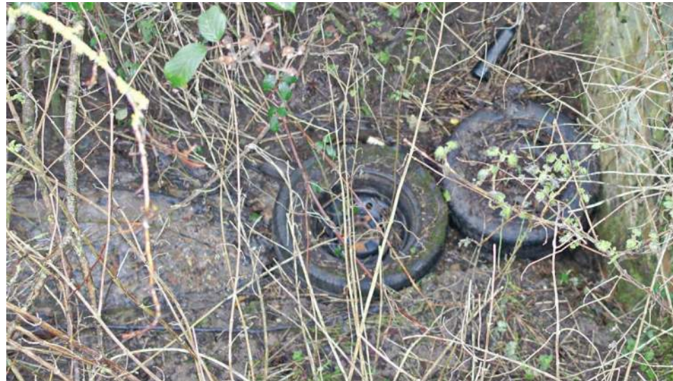
High St East Tires blocking ditch
