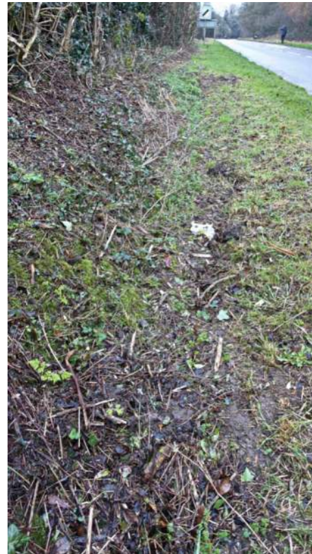
High St West South Overgrown ditch (New Estate)
