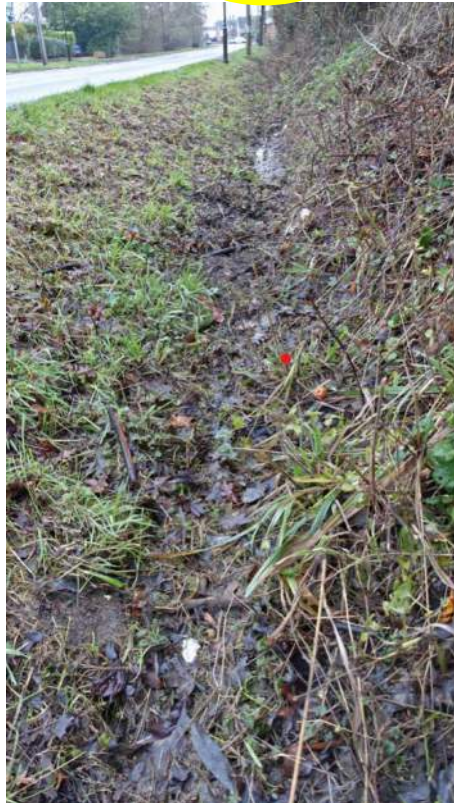
High St West North Overgrown ditch (New Estate)
