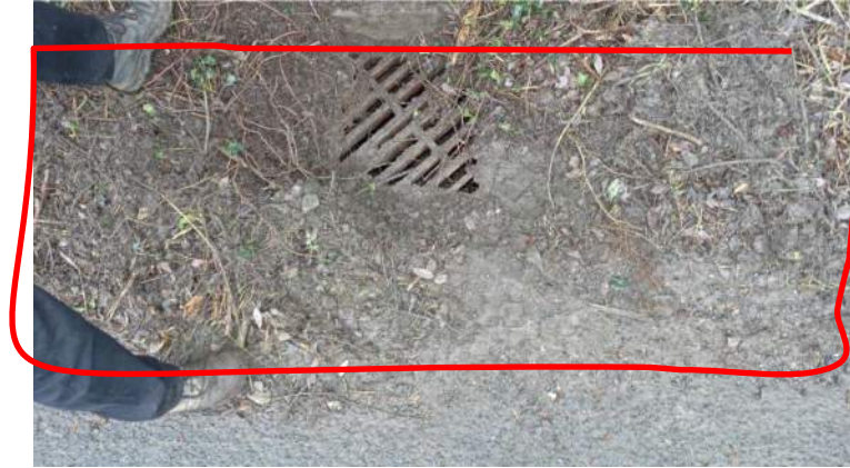
High St West Recovered Kerbside Recovered Road Drain Overgrown Vegetation
