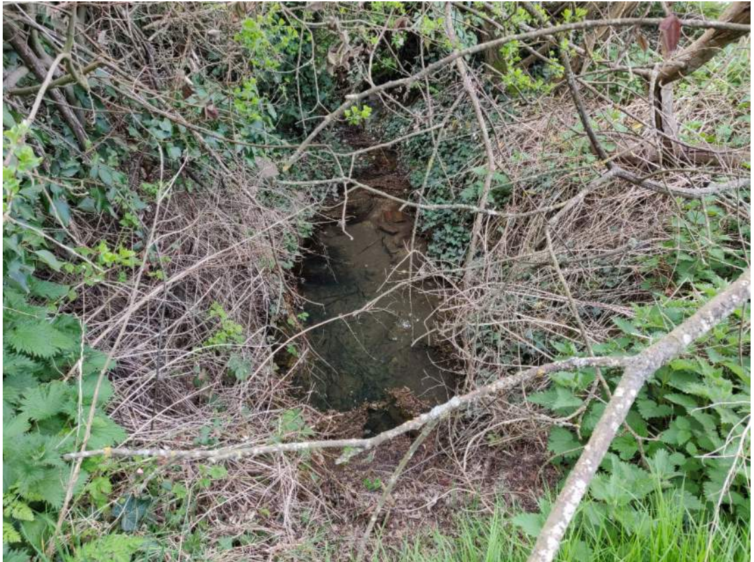
Figure 7: High Street Ditch with Standing Water
