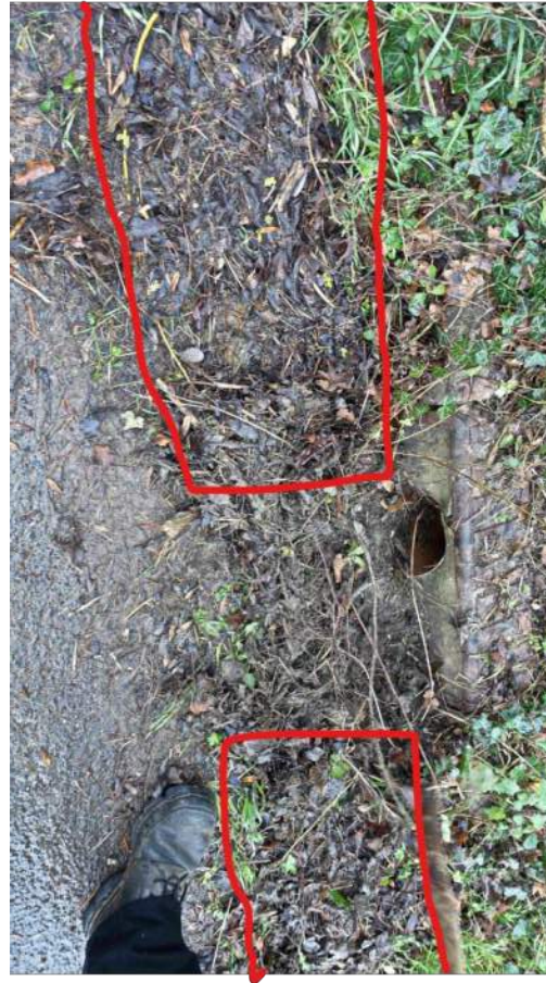
High St East – recovered drain – note overgrown vegetation (>300mm)
