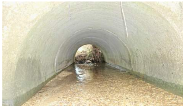
High St East Adjacent to site Sand in drainage tunnel to ditch
