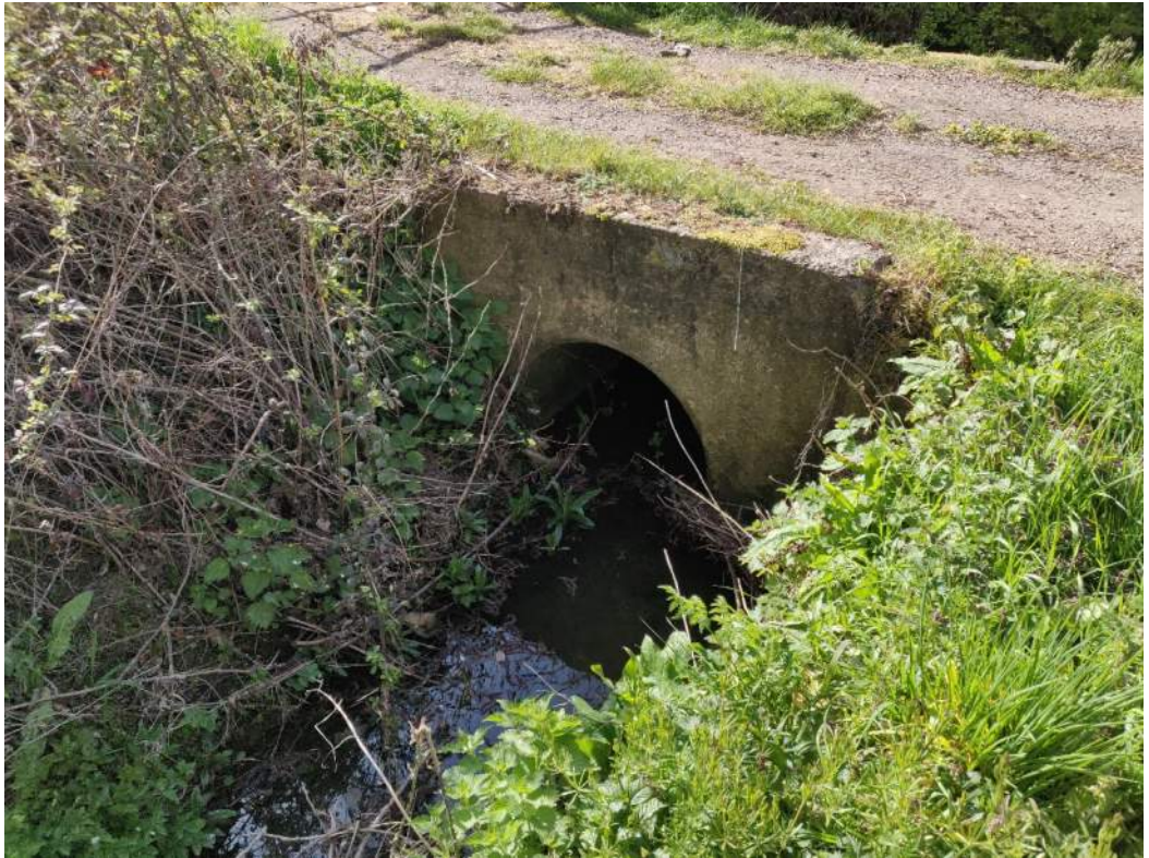
Figure 9: High Street Ditch with Standing Water
