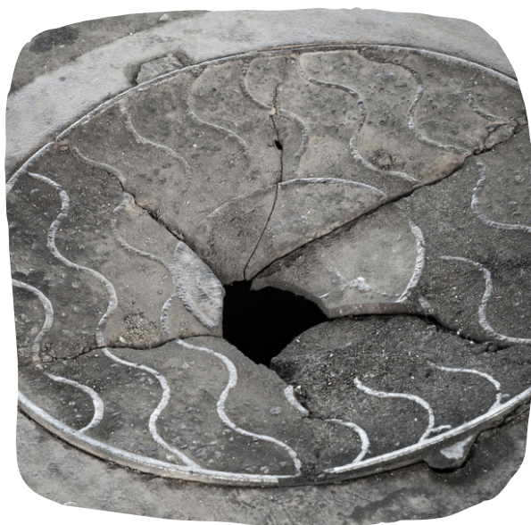
A broken manhole cover in the road.
