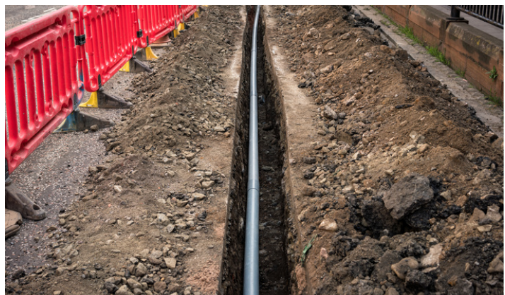
A fibre broadband cable duct being laid in the ground under a footway.
