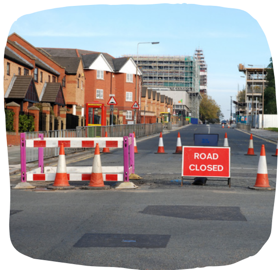
The work site area is cordoned off using safety barriers and cones with a road closed sign to prevent any vehicles using the area.
