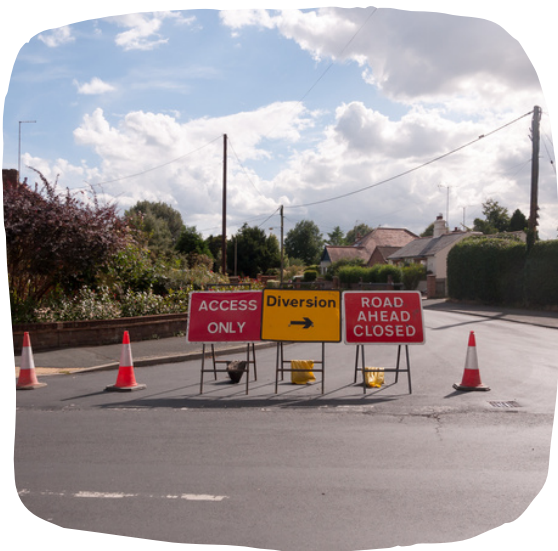
Signs advising motorists to use an alternative designated route (diversion). Only residents of the street may access the road.
