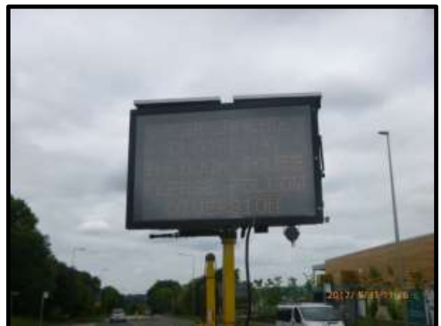
VMS at Newport Road in the traffic island near Saxon Street V7 junction. Newly installed.
