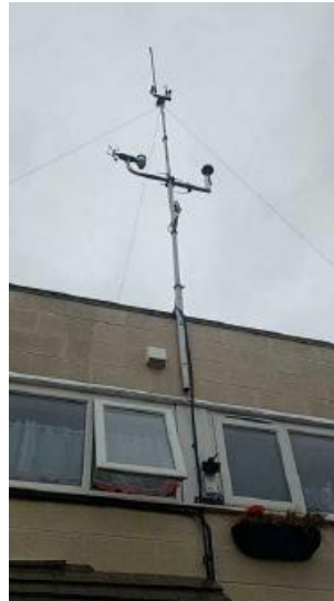
Figure 9 – Example Sensor Installation (Source: Situational Awareness Services Provider)
