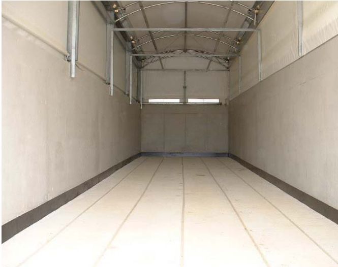
In-vessel composting tunnel
