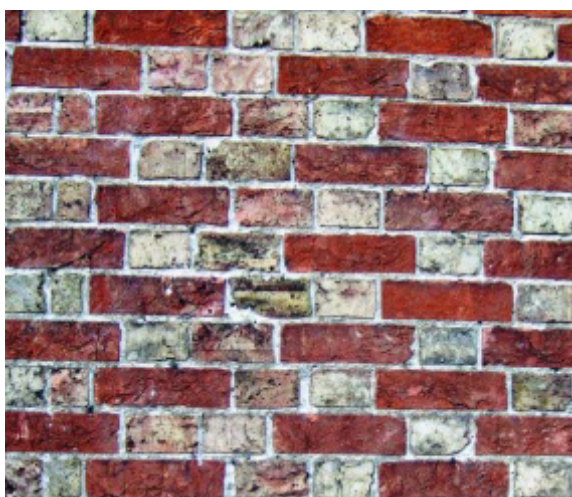
Picture 46 Lime mortar in patterned brickwork. The bond is Flemish diaper-work, made complex by the interleaving of queen closers at the line of connection between two houses.
