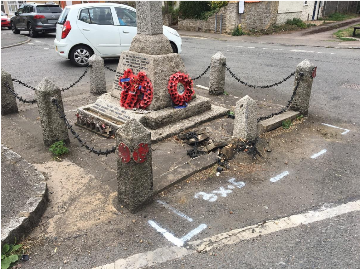
Figure 19: Damage to the War Memorial following a road traffic accident.
