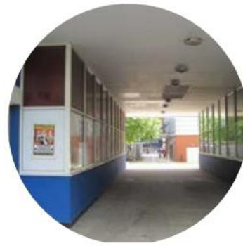
Poor quality pedestrian links and public realm particularly west of the town centre and around Stephenson House.
