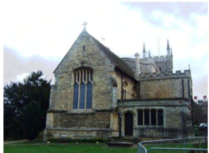
Picture 25 St Peter and St Paul's shows rubble and carved stone used in combination
