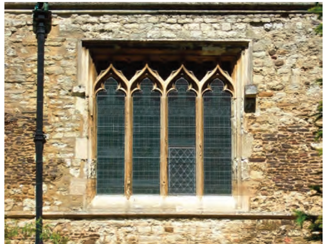
Cusped mullioned window, St Mary's church Bletchley. Note the use of dark brown ironstone in the paler limestone wall. It's presence adds distinctiveness and character.
