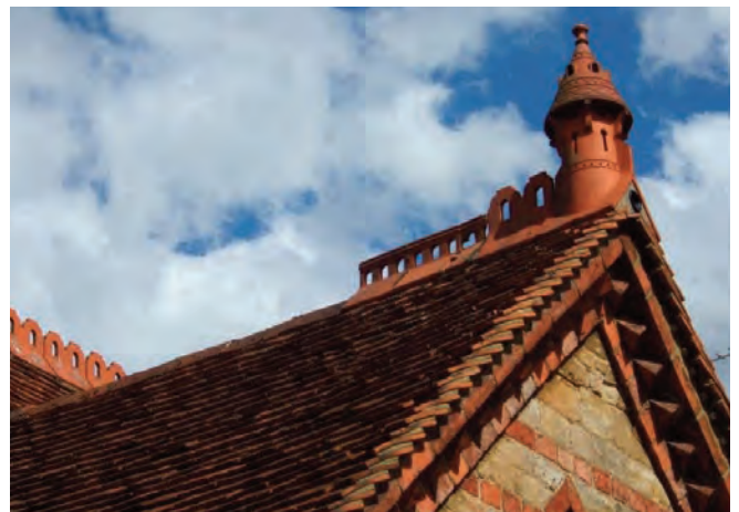
Neatly laid late 19th Century steeply pitched clay tile roof with ornamental ridge tiles and terracotta finial at The Retreat Almshouses off High Street. Note the witch's eye detail at the apex.
