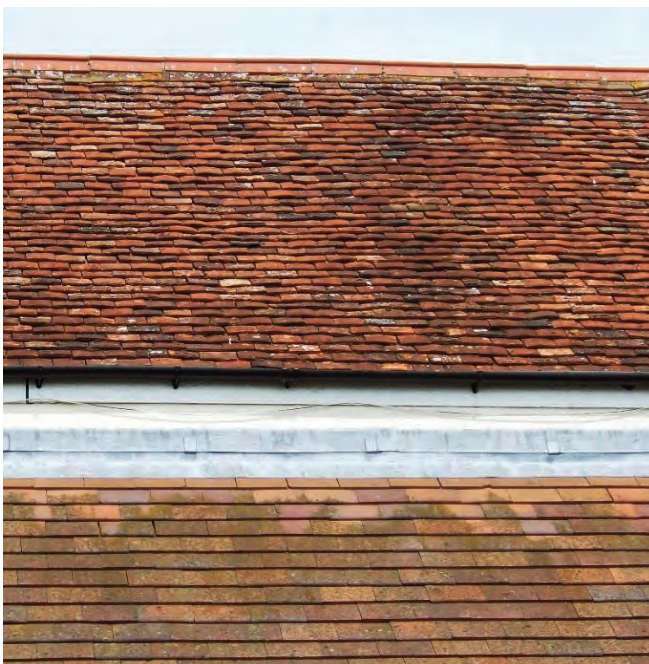
The difference between older handmade tiles and newer machine made tiles is clear when seen side by side. The modern slates lie flatter and have less texture and warmth than the older tiles.
