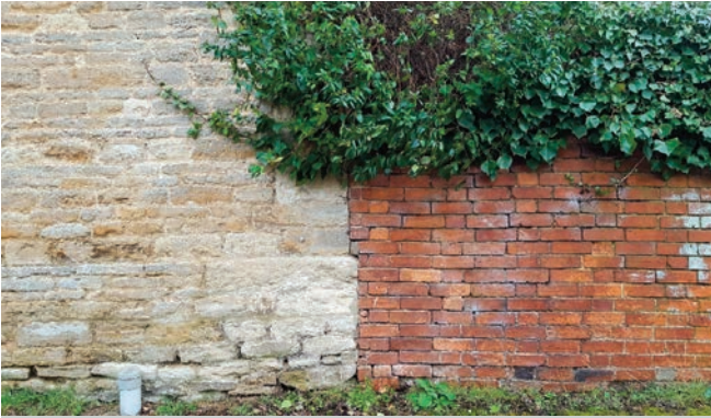
Brook Farmhouse walls - The mellow cream limestone of Brook Farmhouse (GII listed) and soft orange locally made brick in Flemish garden wall bond – three stretchers and a header to each course of bricks – beside Milton Road. It will be important to point the open joints (where the mortar has been flushed out by rain and road splash) in a cement free lime mortar.
