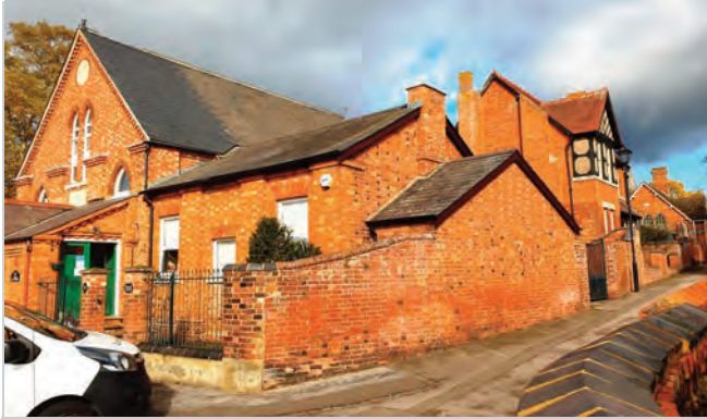
The Wesleyan Chapel and School House. The brickwork is of Flemish bond where headers and stretchers alternate. A chequer board pattern can emerge if alternating colours are used. In the flanking boundary wall and outbuilding the pattern has broken down and appears pockmarked with burnt black headers
