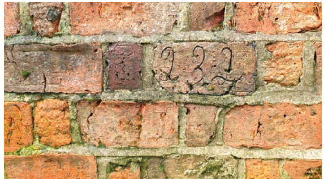
Low brick wall in rat trap bond where the bricks are laid on edge. The meaning of the 232 marking made on the bricks before being kiln fired is not understood at present. The wall has been pointed with a hard cement which is causing the softer brick to flake but the clarity of the numbers is not yet affected
