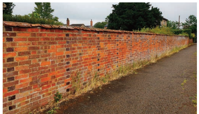
A boundary wall built in Flemish garden wall bond with a pattern formed by inserting a darker brick at every third header on alternating courses
