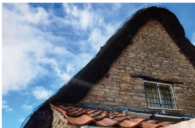
Curved pantiles on a mono-pitch roof next to Horseshoe Cottages with an early metal casement window above
