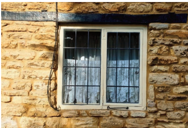
Timber side hung casement window with lead comes under a timber lintel at Horseshoe Cottages. The timber window has pegged mortice and tenon joints and 'HL' hinges and a metal hook window stay
