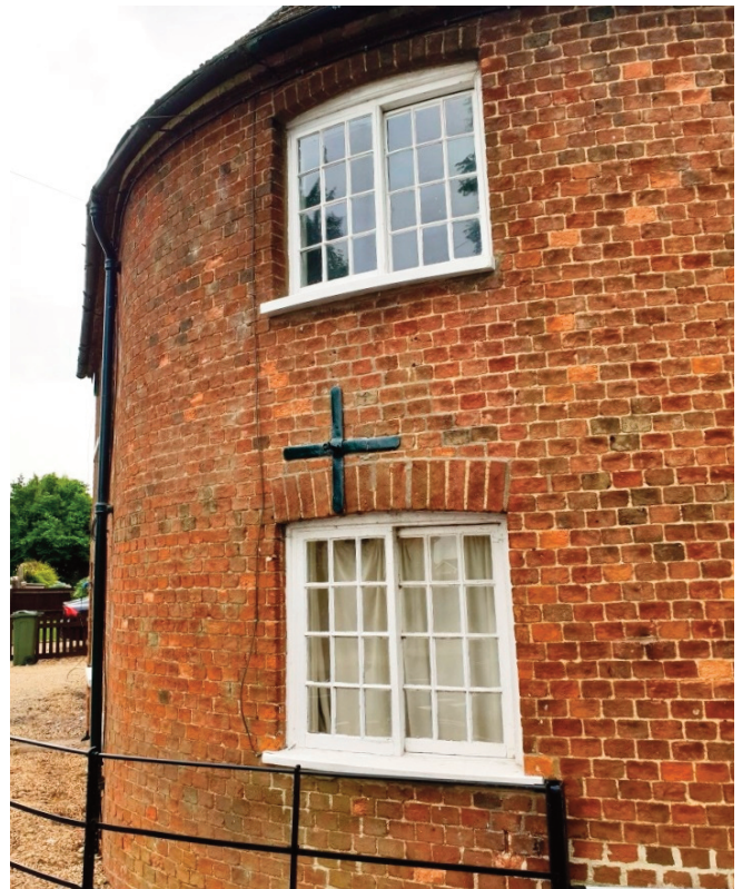
Brick 'headers' used skilfully create a curved wall. The windows are horizontal (Yorkshire) sliding sash that predate vertical sliding sashes. They are of small 12x12 pane puttied into structural (rather than applied) glazing bars under simple segmental brick arches. Some old glass survives and the impressions for a hinge that supported a shutter are still observable.
