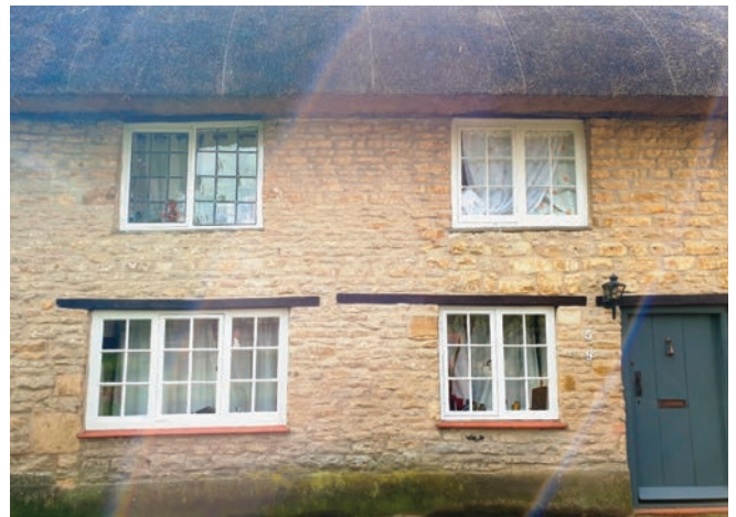
Casement windows; the upper floor has cillless openings and small panes subdivided by lead comes. The glass is not smooth and, in the ground floor timber windows, is puttied into structural (rather than applied) glazing bars. Some windows on the ground floor retain evidence of shutters that have now been removed. The door is a simple plank door with brass knocker and a latch
