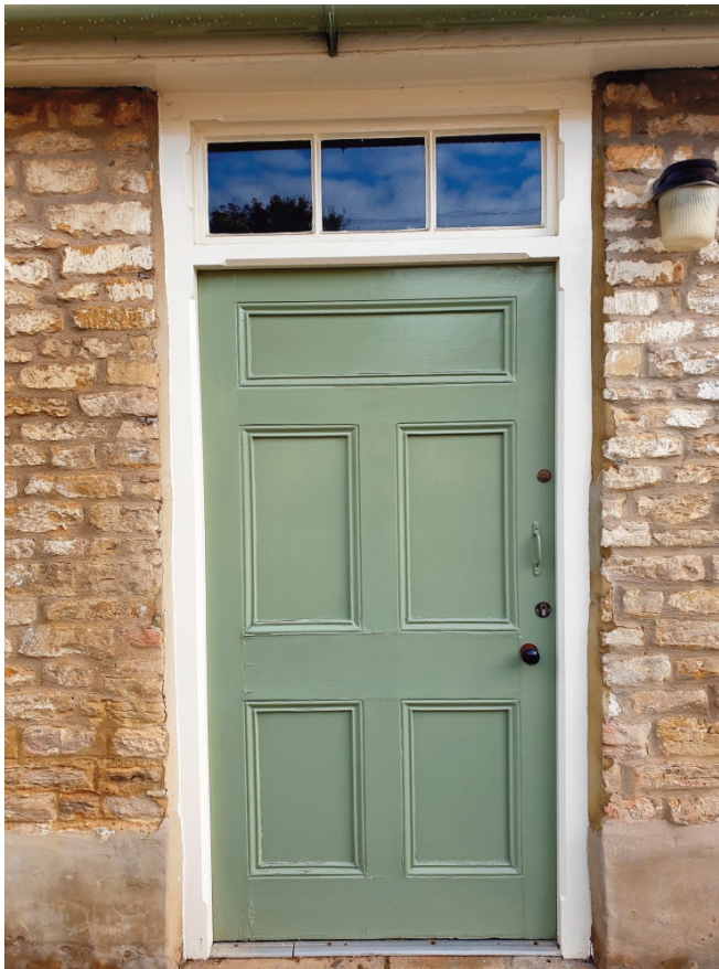
Late Victorian door and frame, note fanlight and the simple chamfer detail to the frame. The knocker and letter box are missing as this is the door to the village reading room rather than a domestic dwelling
