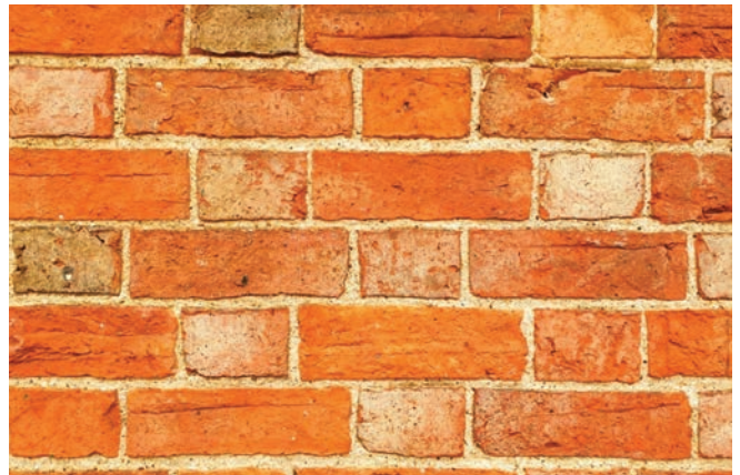
Brickwork, the lime mortar has been yellowed by the choice and amount of sandy aggregate
