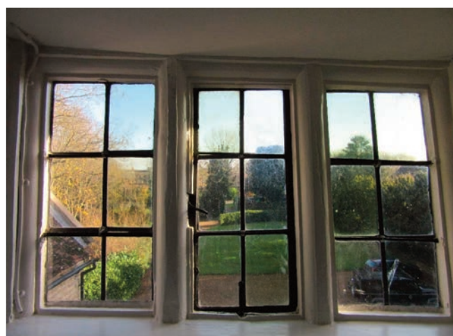
Uneven glazing in a C17th mullion window.
