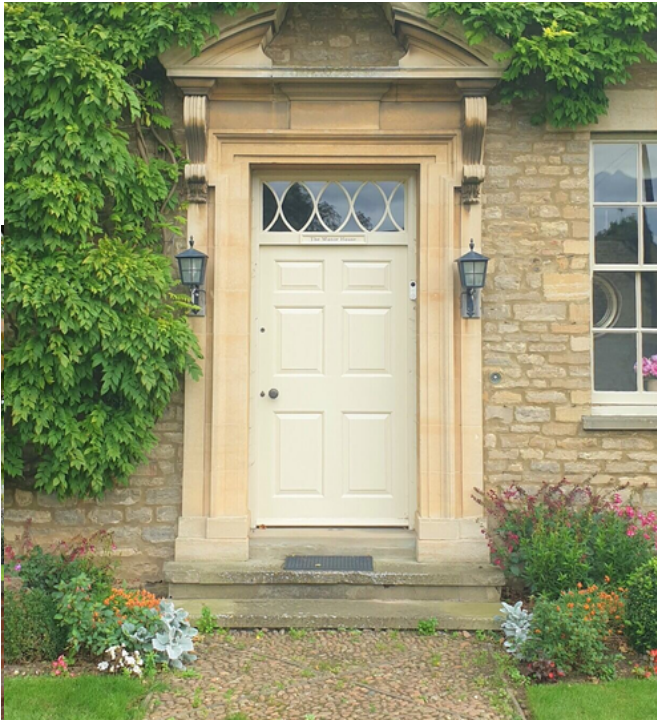
Door at The Manor House, High Street. The house has origins in the C17th; this is a 6-panel door divided by a horizontal frieze rail and a locking rail and then divided vertically by central 'muntin' boards. There is a shouldered stone door surround, itself contained within shallow pilasters, topped by fluted consoled brackets supporting a broken segmental pediment above sitting on plinth. The ornate glazed fan or transom light is above the door. The door itself is only occupies a relatively modest proportion of this grand composition.
