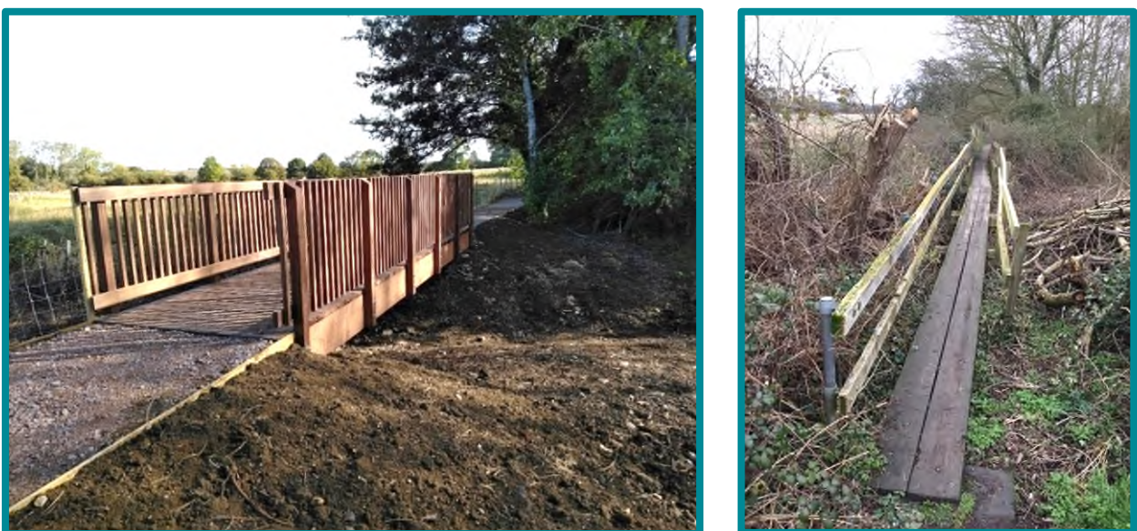
Figure 16. A newly installed bridge and approach (left) on Newport Pagnell Footpath 15 with improved accessibility to the original narrow structure (right)
