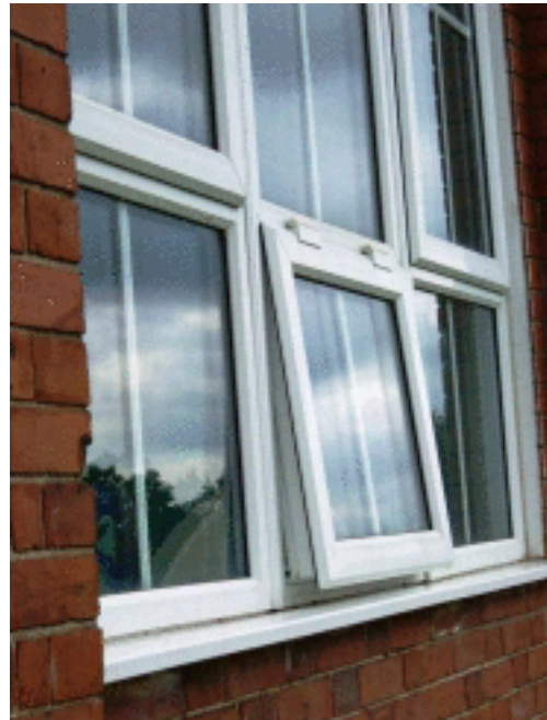
Picture 3.7 Ungainly plastic windows with protruding casements, mitred joints and polythene finish are a conspicuous and discordant alternative to timber. Their medium to long term benefits are increasingly called into question
