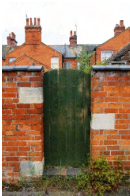
Picture 2.88 Typical rear gate arrangement.
