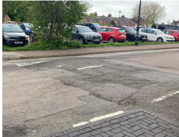
Figure 30: A well-worn road hump.
