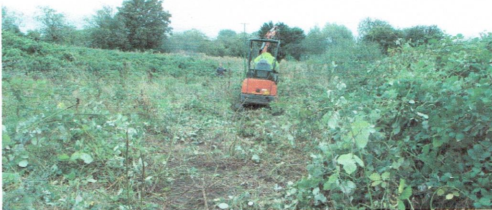
Photo No.1 Small excavator with figure guiding some metres below. The use of this small machine was slow and hazardous due to the ruts.
