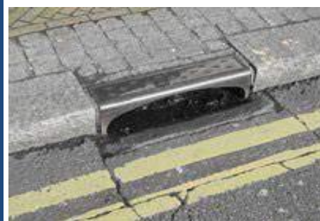
Typical cast iron Kerb Weir within kerb line
