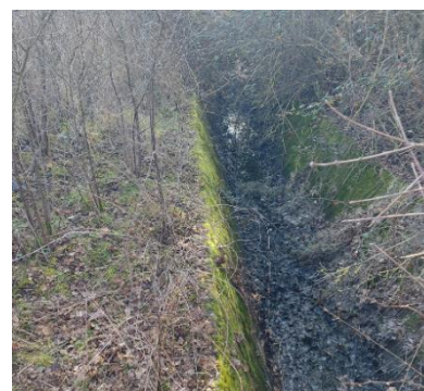
Channelised Concrete Ditch on the A4146
