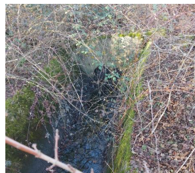
Channelised Concrete Ditch on the A4146
