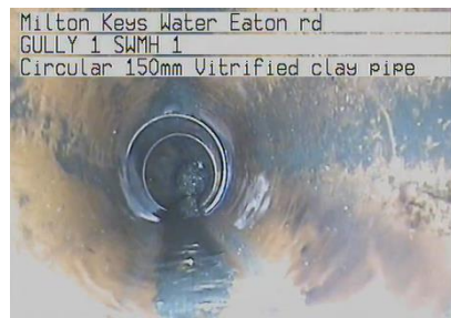
E.g., Water Eaton Road 150mm clay pipe
