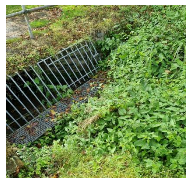
E.g., Trash Grill – Before cleaning
