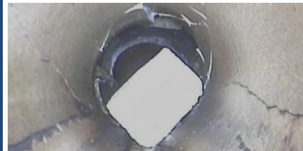
E.g., Blockage in pipe due to Brick in pipe and pipe cracking
