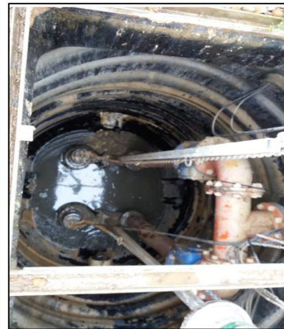
E.g., Pump station Wet well with Two pumps stationed in bottom of chamber
