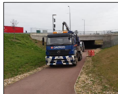
E.g., Tanker cleaning and jetting chamber to remove silt build up
